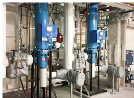
Steam, Hot water
