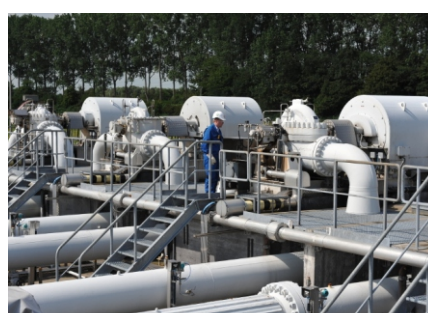
Power Pump Station
